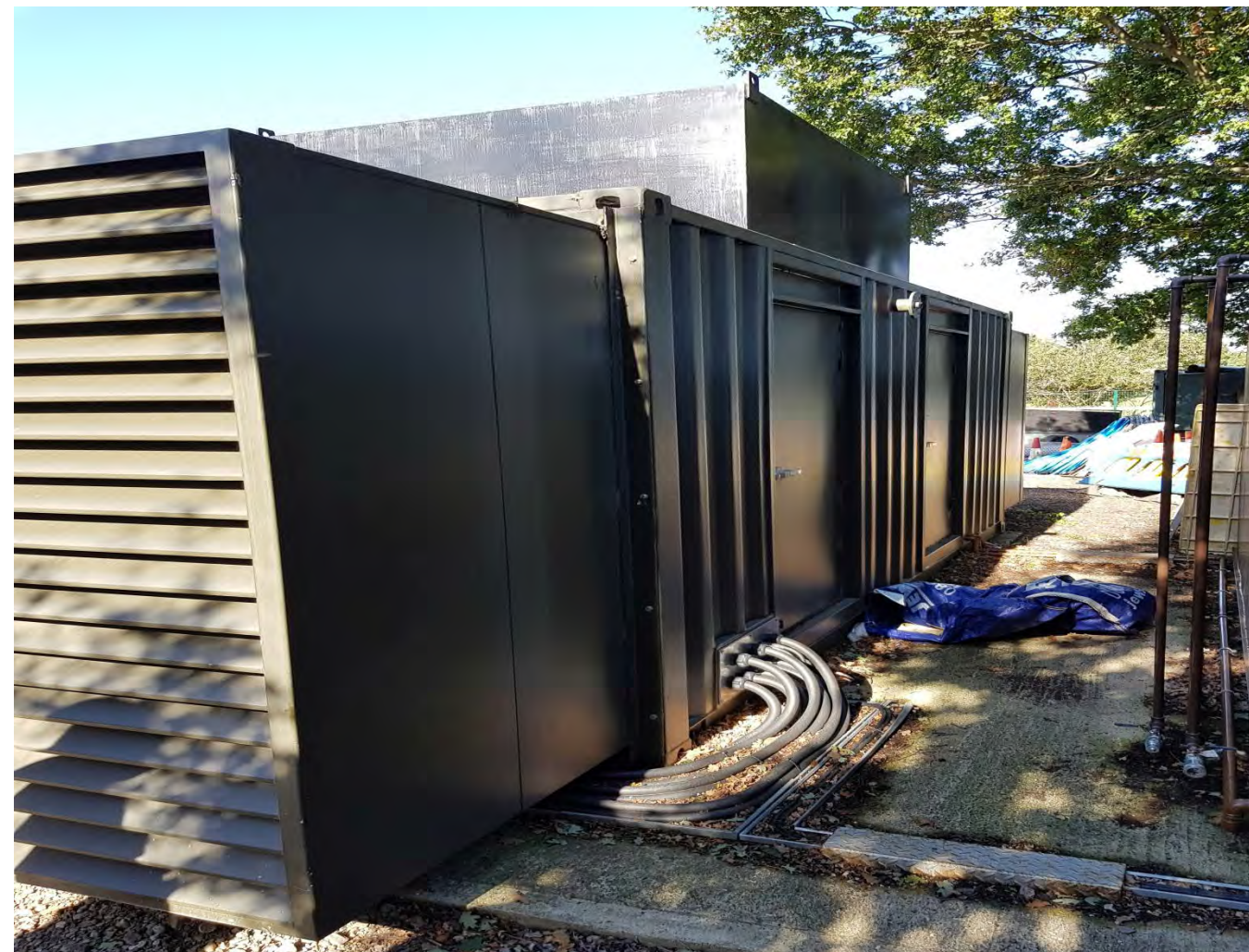
Figure 10: Existing 800 kVA containerised emergency standby generator set at Substation A
