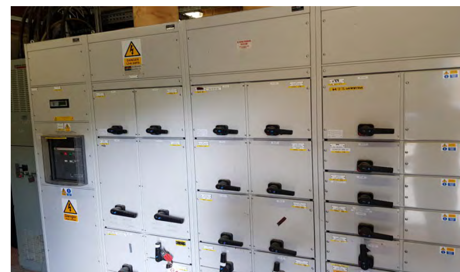
Figure 6: Existing 1600A Dorman Smith LV Switchboard
